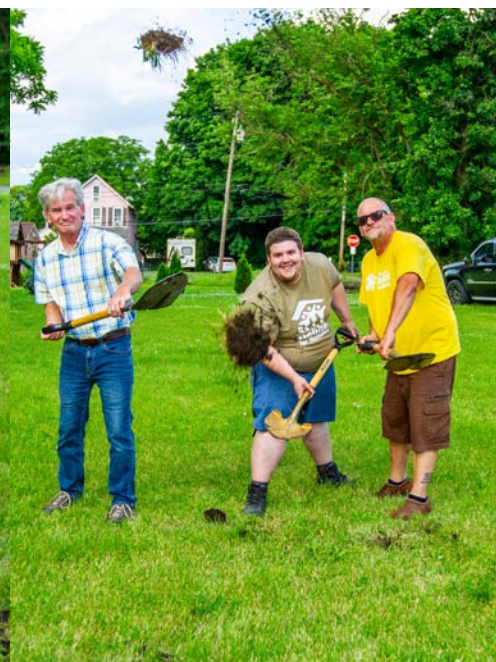
(From left to right): Chris Motzenbecker, Warren County Habitat Construction Supervisor, Matthew Chobot and Michael “Scrappy” Chobot dig the first holes on the land that will soon become their home.
